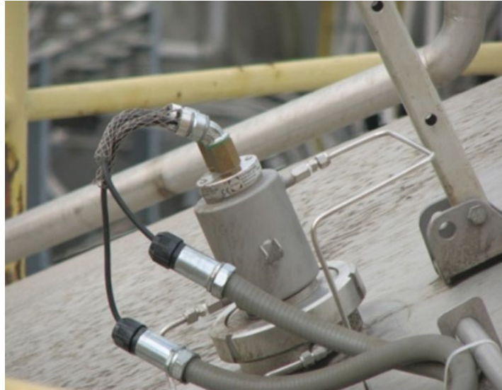
Figure 3. Camera installed in an air-cooled housing.
